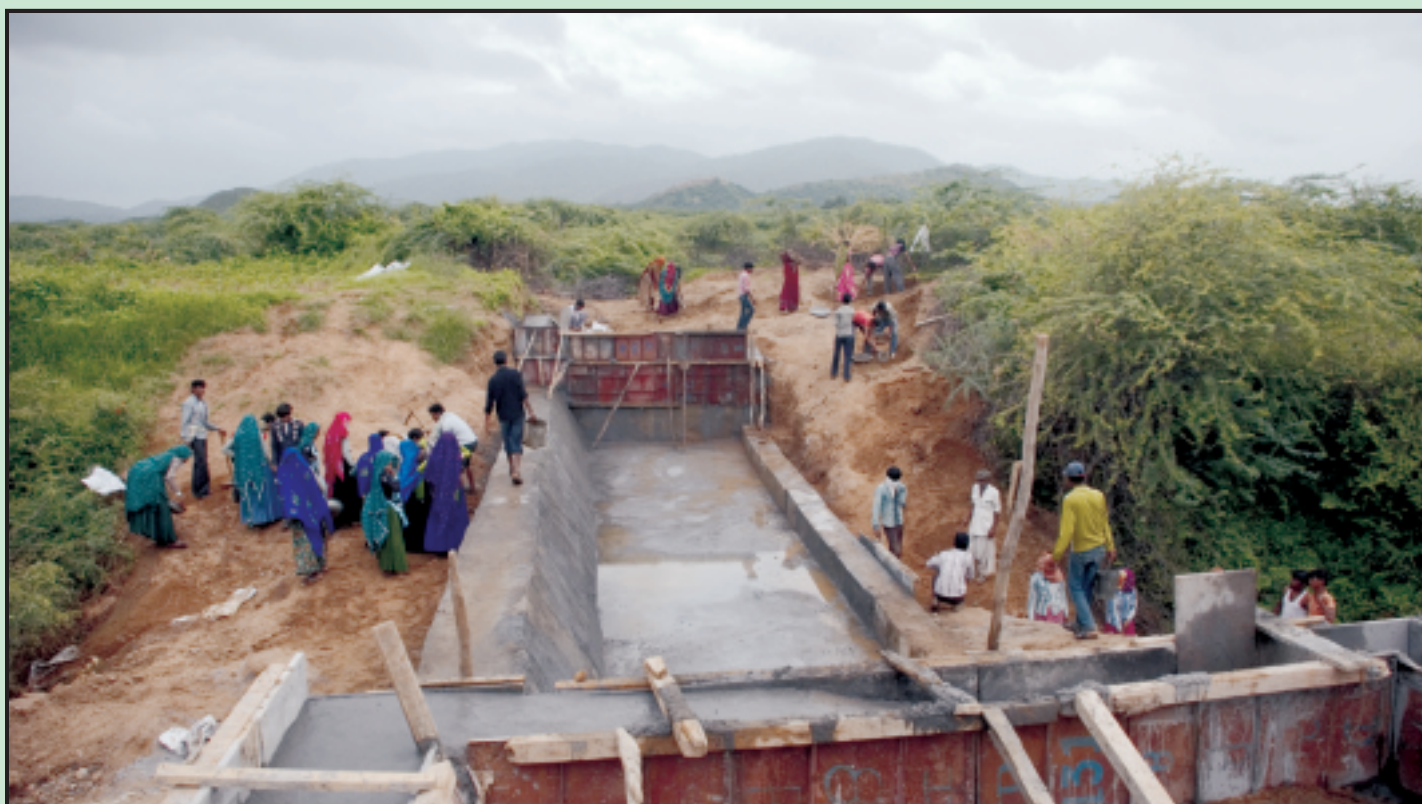
Check Dam Construction Under Mgnrega in Village Nichala Bandh, Block Amirgarh, District Banaskantha, Gujarat
