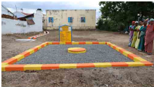
Erode District - Anthiyur Block - Brammadesam panchayat MGNREGS 2018 -19 Community Soak Pit - Vertical Estimate Amount - 1.16Lakhs
