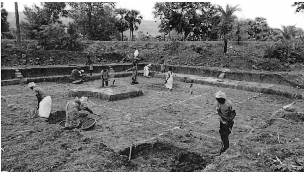
Self-help group mates supervising construction of a dobha in Hethbandha, Boarijore (Godda)
